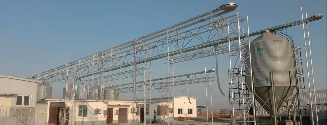
T160 central filling line for 24000 finisher farm
